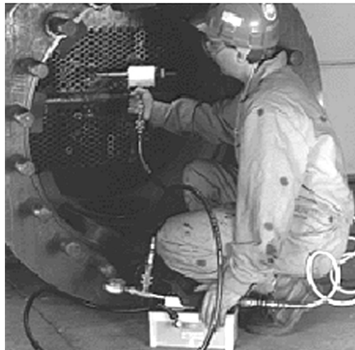
Fig. 3 Typical Installation of Mechanical Fit Tube Plugs (©2006 Photo courtesy of EST Group Inc., used with permission.)
