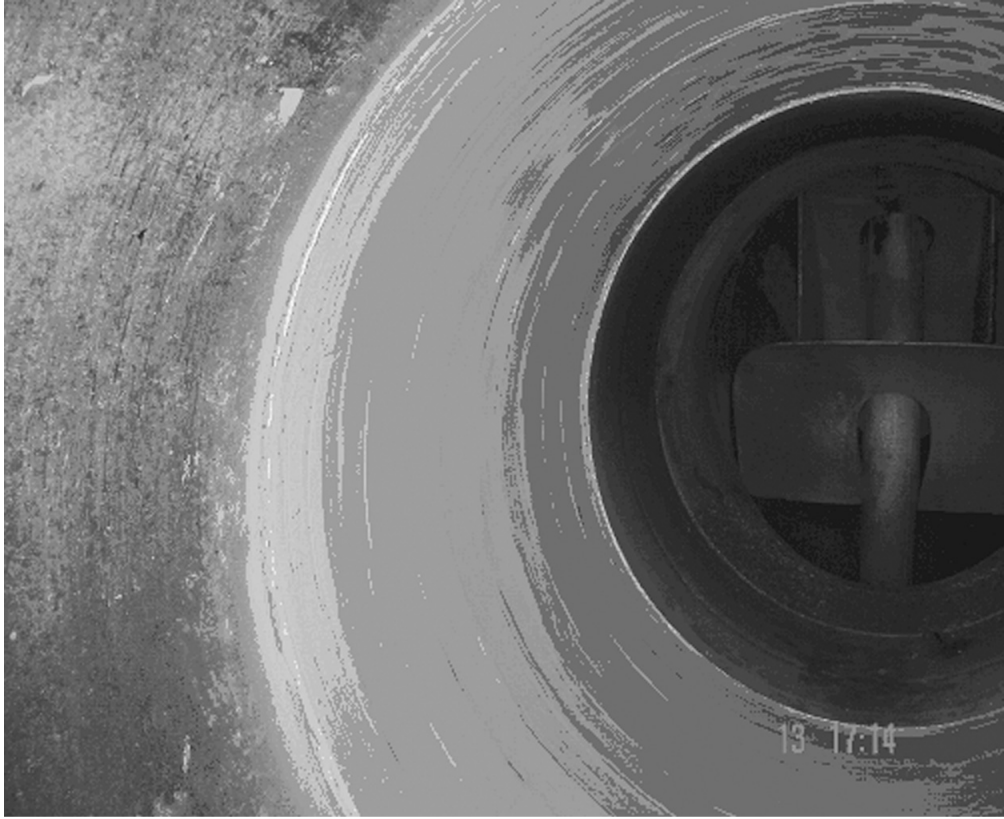
Fig. 1 Structural Liner in Raw Water System
